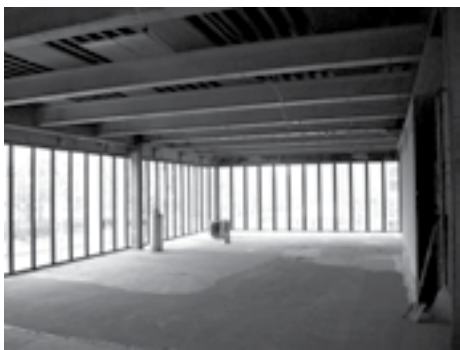
Interior demolition is nearly complete at NJSBA Headquarters at 413 W. State St..
